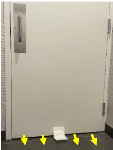
Figure 3. View from inside a negative pressure room.
